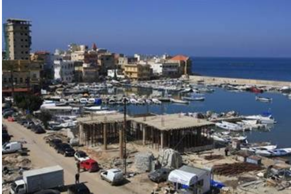
The new structure is taking shape at Tyre’s port.(The Daily Star/ Mohammad Zaatari)
